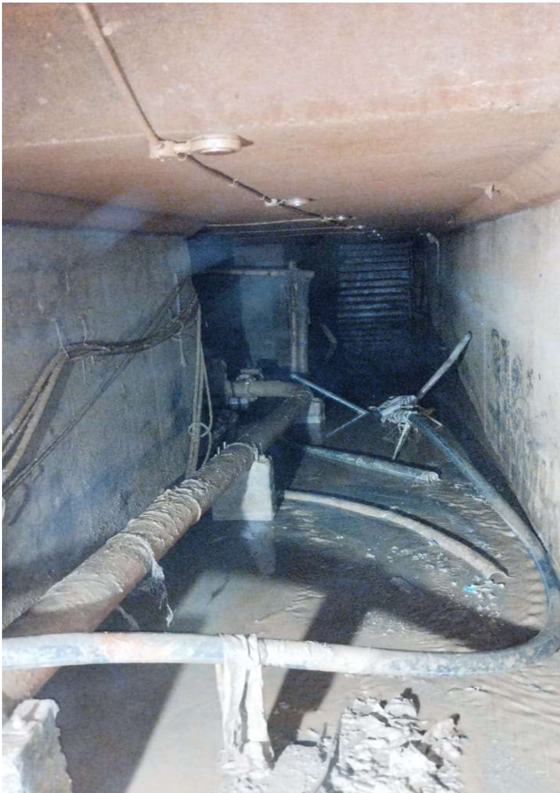
Existing dewatering pipeline inside Dam gallery
